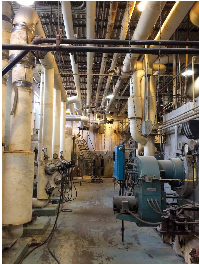
FIGURE 14. Biomass Main Boiler.
