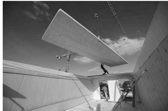
FIGURE 10. Image of on site assembly of stacked board ceiling elements (photo: KLH Austria).
